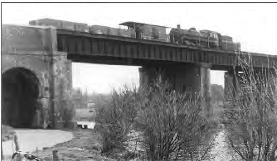
River Stour Bridge at Wimborne, looking south, Spring 1967, with a BR 76XXX 2-6-0 shunting the yard. S&D trains ran over this bridge from Wimborne Junction to the station, between 1860 and 1933. The state of the bridge was used as a reason for final closure of the remaining line from Poole in 1977. Peter Russell
