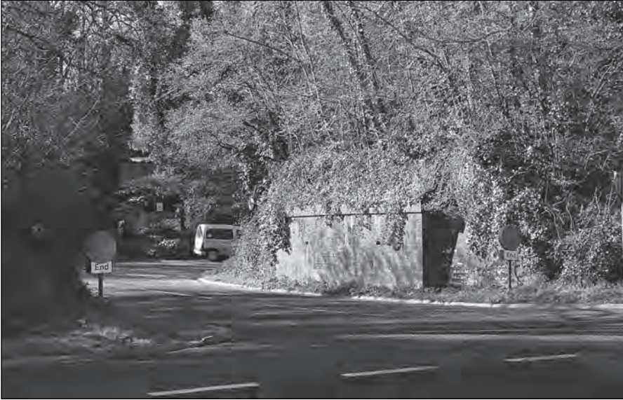
The remaining (west) wall of Digger's Bridge, looking SE, April 10th 2008. This bridge once carried the S&D's Wimborne loop over Candy's Lane between Corfe Mullen Junction and Carter's Siding (off left). The cut-off to Broadstone ran on the skyline among the trees in the background, Goodchild's Bridge being on a direct line from the camera through the entry from the A31 (foreground). Peter Russell
