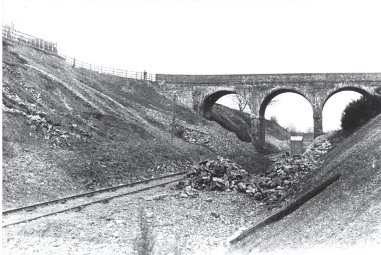
As evidenced here, the deep cutting near the summit of the 'cut-off' was prone to slippage. The 1925 plan included the provision of additional drainage and a retaining wall on the Down side at this location (on the right of the picture). Ashington Lane Bridge (No. 238) is prominent in the background. [Unconfirmed photographer, possibly T E Maidment; undated, circa 1890-1900, S&DRT collection ref. WSHSD_P301_038.]
